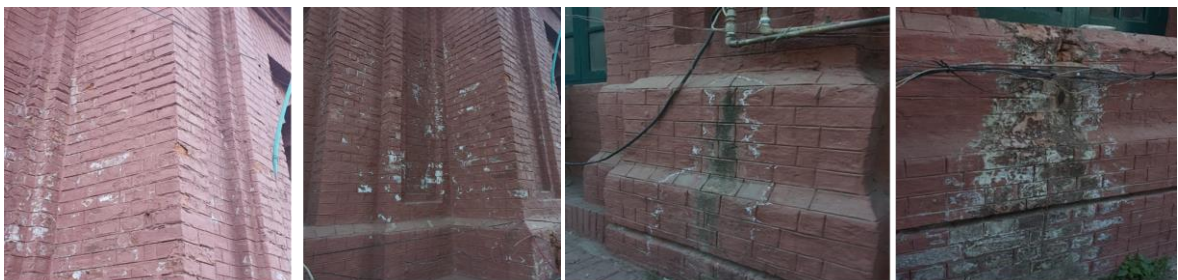
Figure 18: Efflorescence has damaged the outer surfaces
