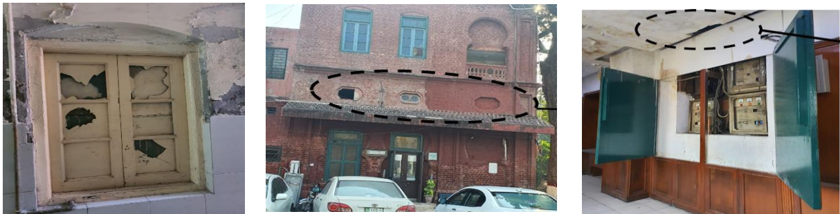
Figure 20: Lack of maintenance can harm structure more than any other agent
