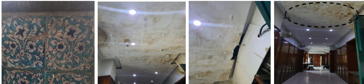
Figure 19: Seepage has destroyed the internal surfaces
